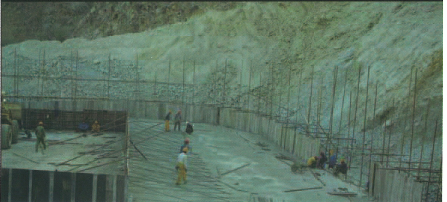
Construction in progress in the mine site. Production to start end of 2009.
